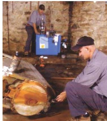
Haldeman Mechanical employees Tavi Nistor (foreground) and Bill Aller prepare to remove the 44-year-old boiler.
